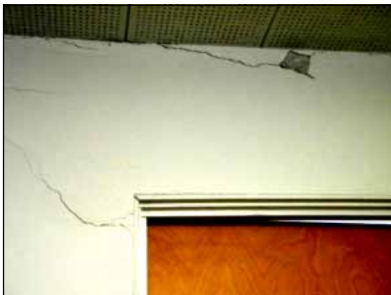
The cracks are bad ...
